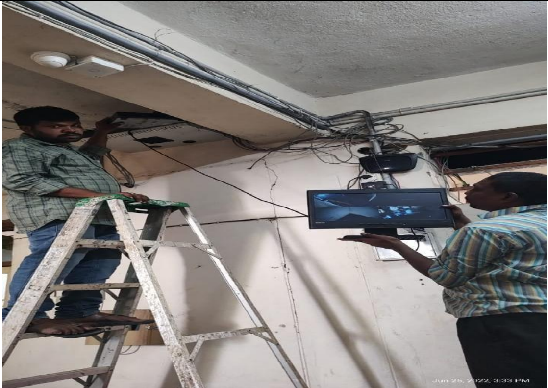
CC- Camera Maintenance
