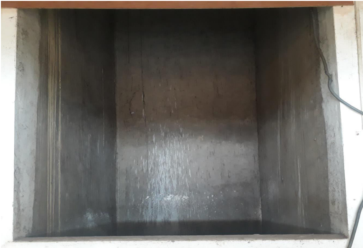
Provision for Lift
